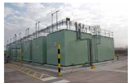
Tank Farm at the new Certas Energy's new distribution centre in Yelland, North Devon.
